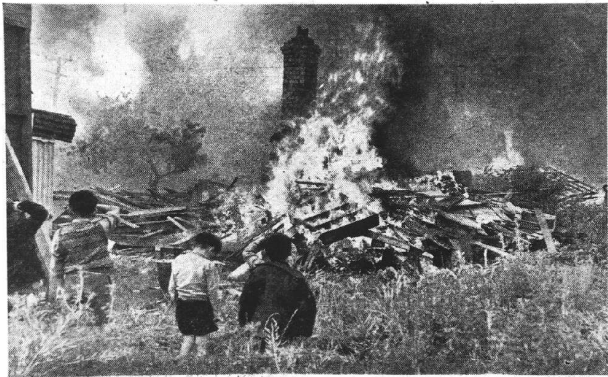
One of the ramshackle homes at Orakei set on fire after demolition yesterday.
